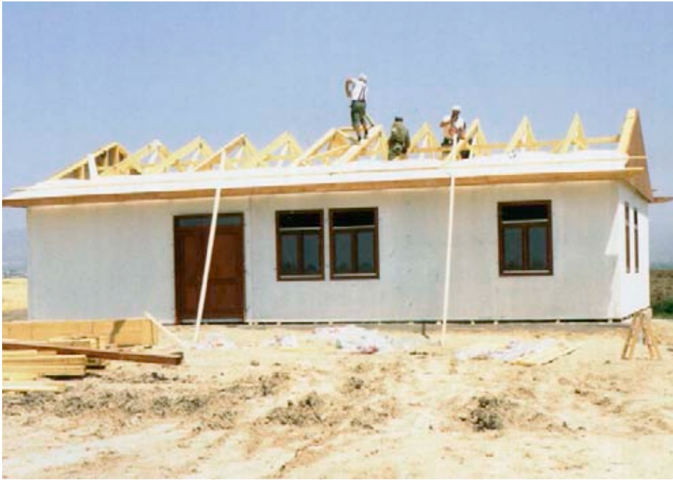
Energy and determination: with support from Diakonie Katastrophenhilfe over 200 prefabricated houses were built in Armenia.
