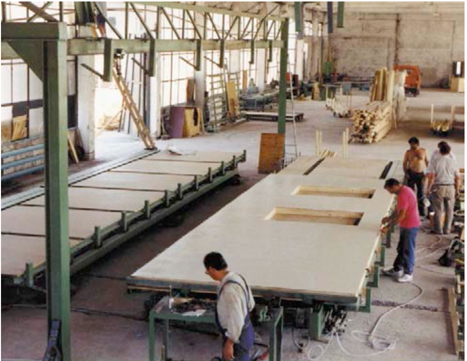
Uncomplicated ideas: after the earthquake in Armenia Diakonie Katastrophenhilfe sets up a factory for prefabricated houses at the location.
