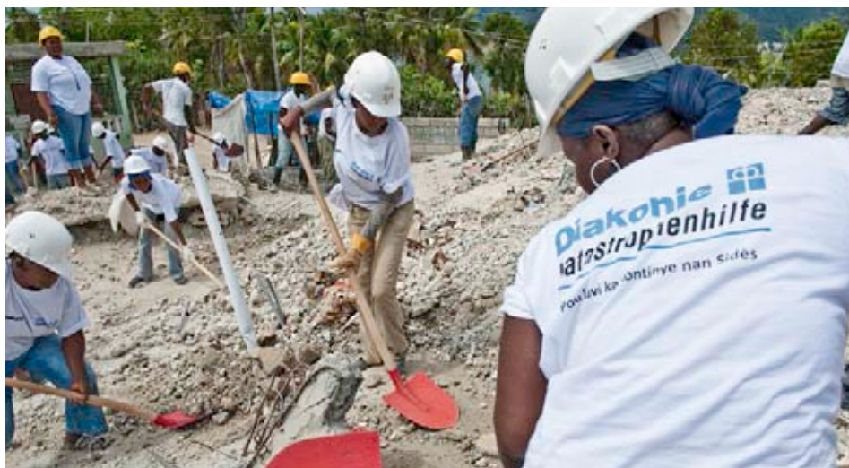
After the devastating earthquake on Haiti in 2010, a “Cash-for-work” project helped to clear away the rubble and debris.
