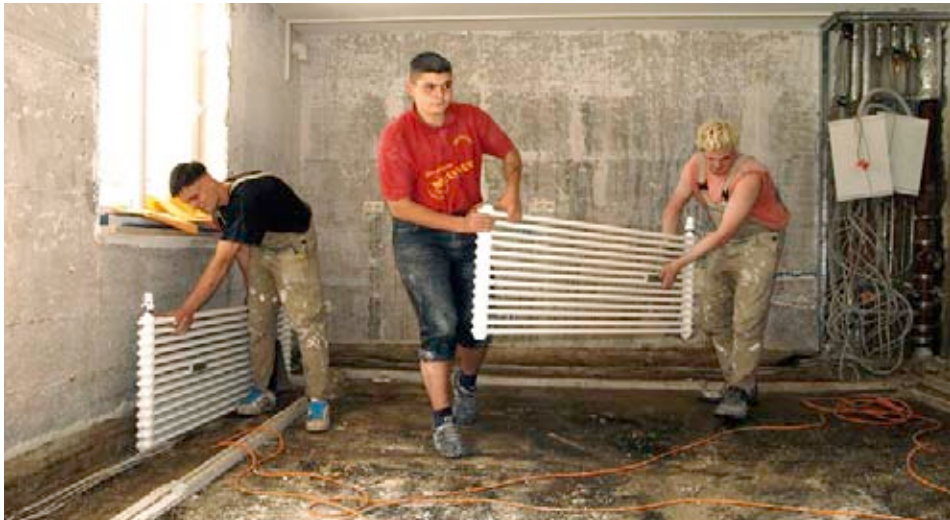
After the flood: in Pirna a house has to be refurbished after the flood in 2002.
