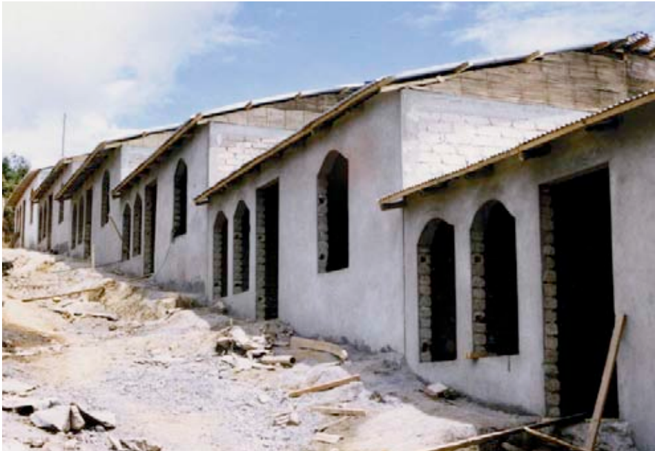
After the earthquake in Colombia Diakonie Katastrophenhilfe facilitates a comprehensive reconstruction programme.
